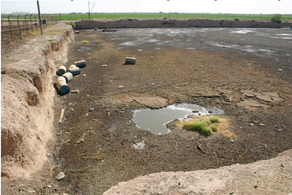
Figure 6 Anaerobic Lagoon with crust showing methane gas breakthrough
